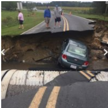
A sinkhole opened up on Ticker Rd in Sampson County. Photo taken by WNCT via WNCN
