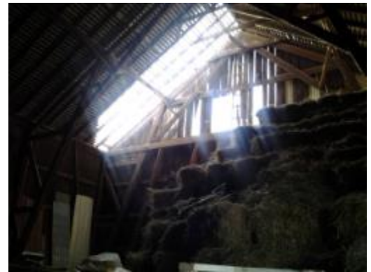
Figure 2: Barn with Roof Damage
