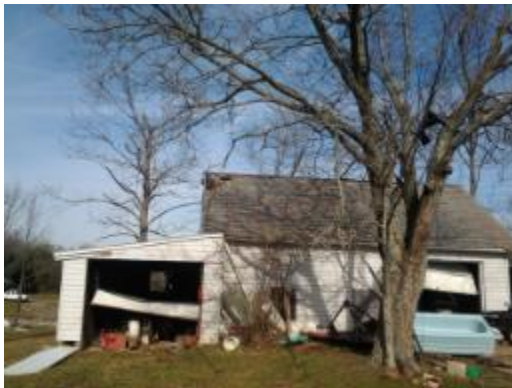
Figure 3: Old Barn Moved Several Inches off its Foundation When the Winds Knocked in the Garage Doors.
