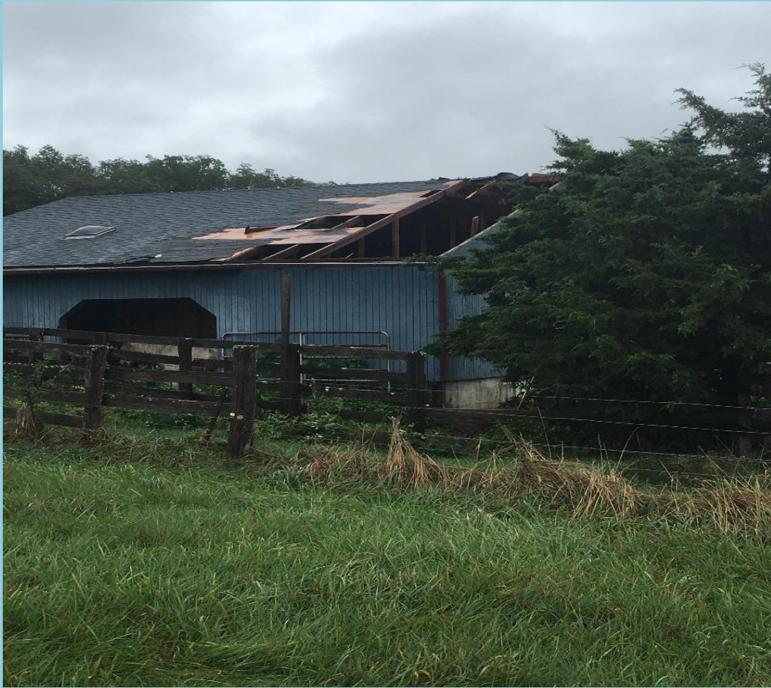
Figure 2. Barn damage from EF-1 tornado near Dove Drive.
